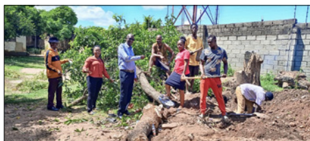
The construction of Chipata South Parish School in Zambia was made possible with financial aid from the Link Parish of Keynsham, which has also donated IT kit. Photo: Diocese of Bath & Wells
