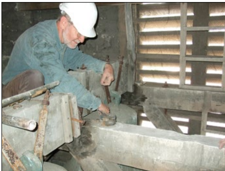
A team of volunteers have made a splendid start on dismantling the old bell installation. Above, Roger Button removes a tie bar.
